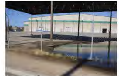
Standing water remains at the vacant tomato cannery multiple days after a rain event, showing the need for stormwater management.
